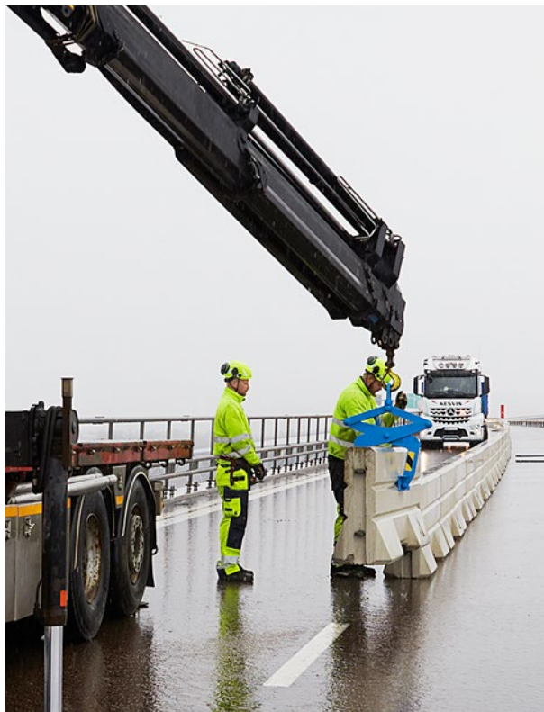
All the way from planning to the practical work out at work sites, Ramudden focuses on safety and efficiency.
